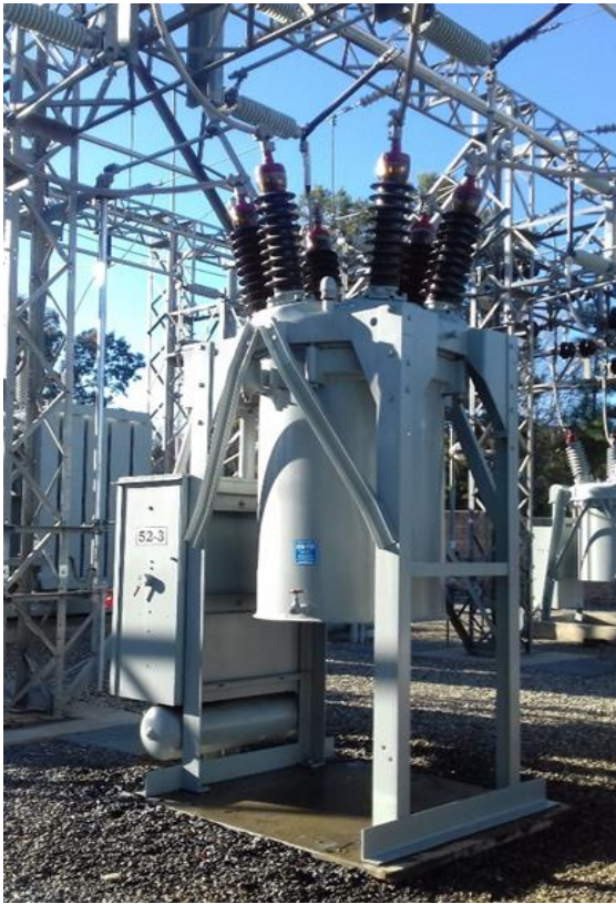
Typical Oil Circuit Breaker (Aged Unit)
