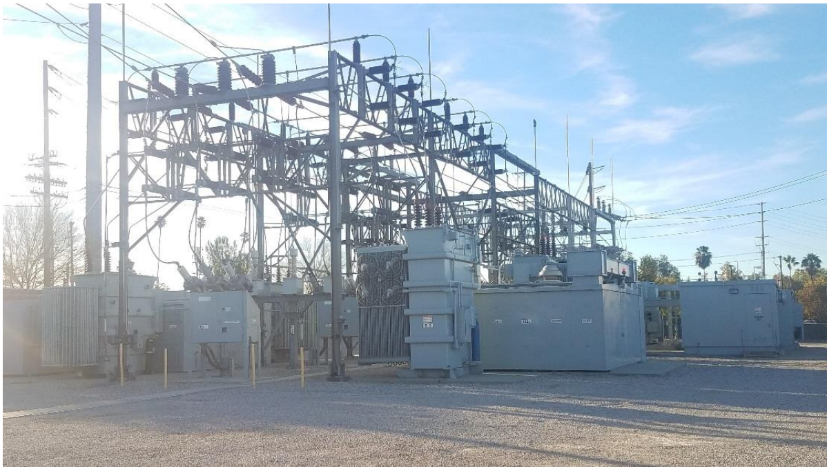
Existing High Profile Hunter Substation
