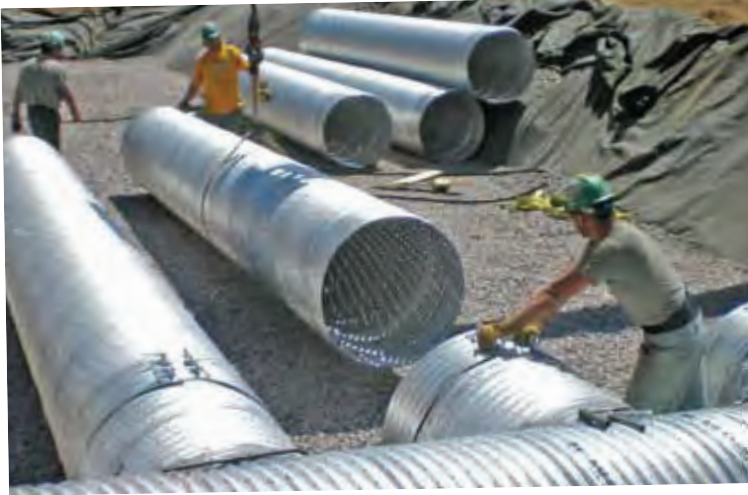
Perforated CMP infiltration system
