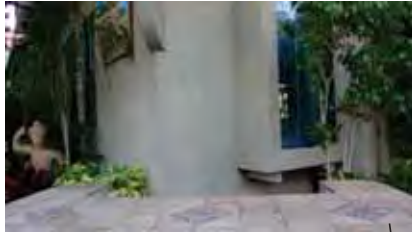
Proposing removal of service station to gain access to window, which will become our entry door
