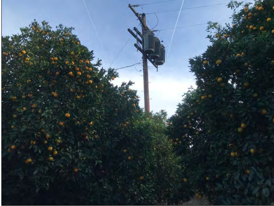
Photo 9: View of pole-mounted transformers.
