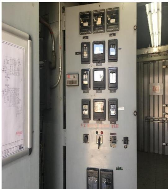
Electromechanical Relays at Freeman
