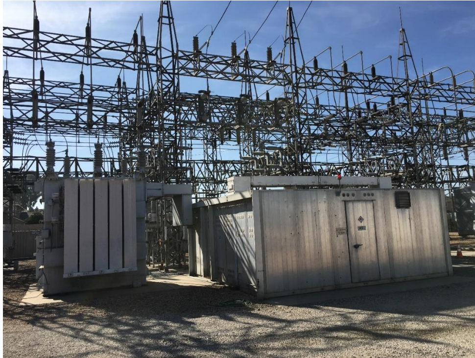
Freeman Switchgear 1 & 2 and Substation Power Transformer
