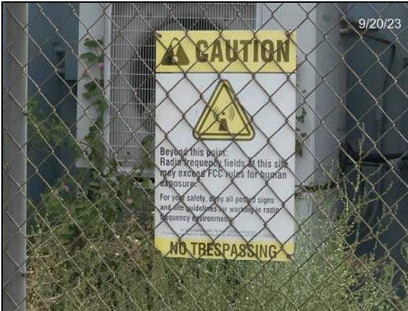
5. T-Mobile Perimeter Signage
