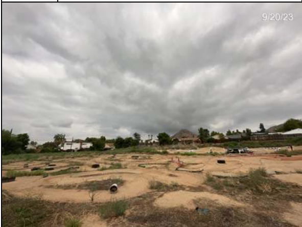
12. AT&T Broadcast North
