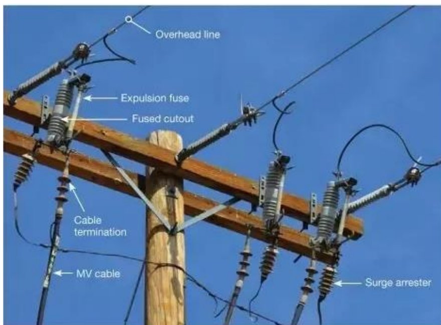
Fused Cutouts on Crossarm
