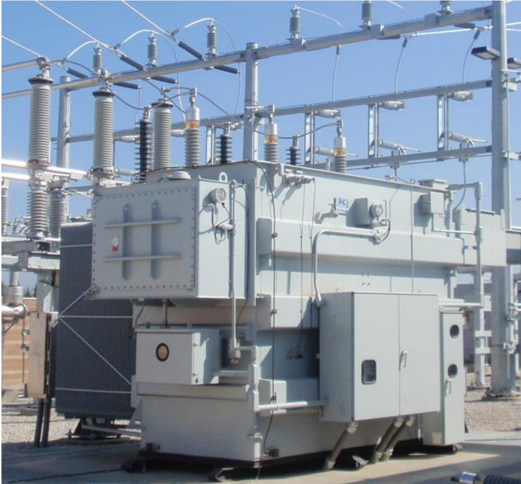
Typical Substation Power Transformer
