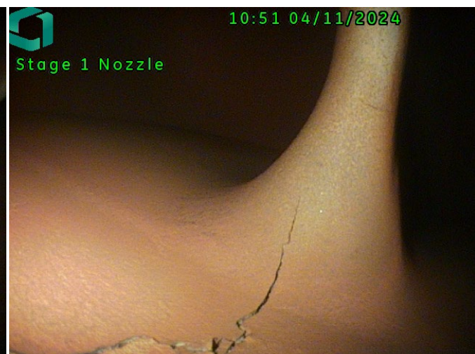
Figure 3. Stage one nozzle - flume crack
