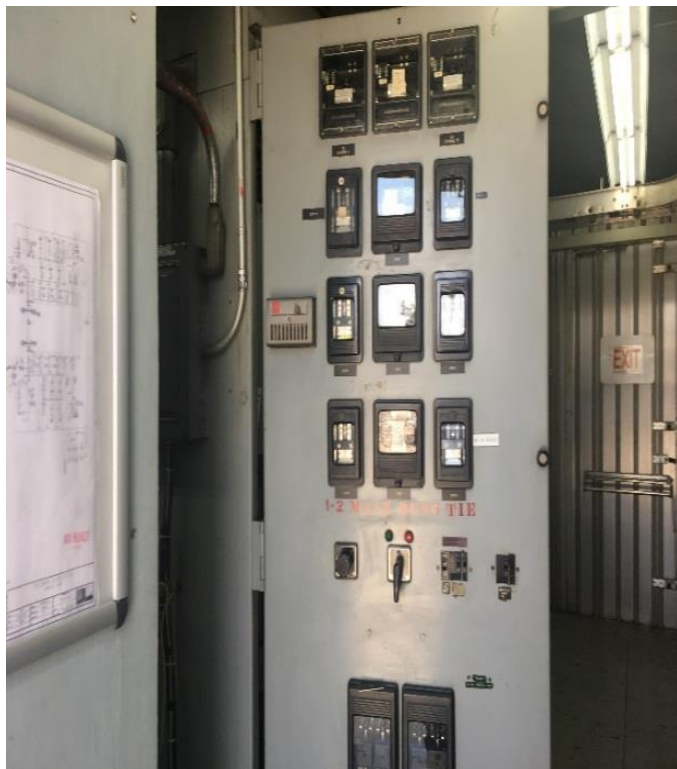
Typical 1 st Generation Digital Relays
