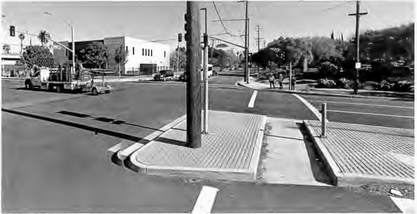
Intersection 19 – Magnolia Ave & Polk St - Looking southbound. Improvements include – high visibility crosswalks & audible pedestrian pushbuttons. Note extra ped button at median refuge island. Adjacent to Kaiser Hospital (Top picture)
