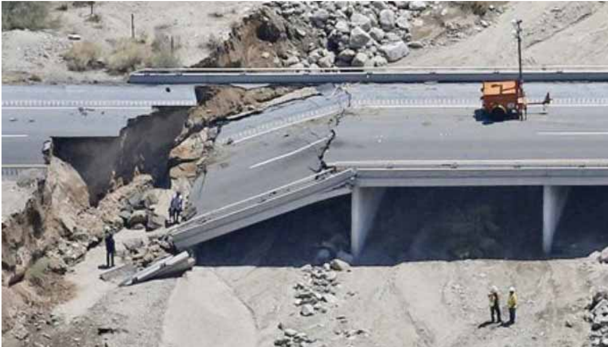
Bridge washout along I-10 near Desert Center, July 2015.
