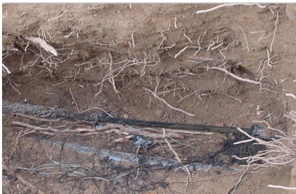
Aged Underground Infrastructure: Cable-in-Conduit System
