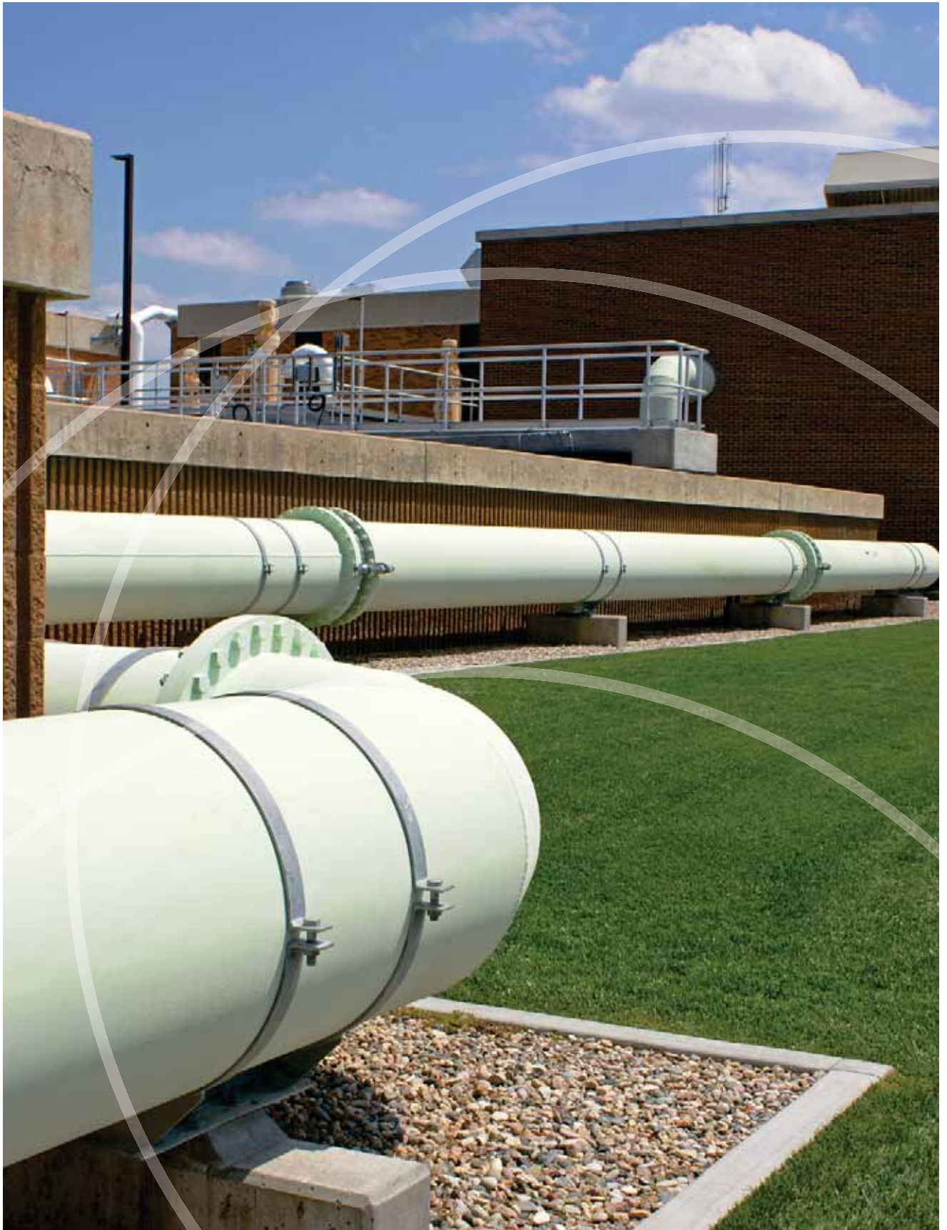
The Drake Water Reclamation Facility has implemented an ISO 14001 certification for its Environmental Management System.
