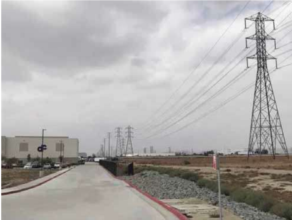
Photo 3: East of Mira Loma Substation.
