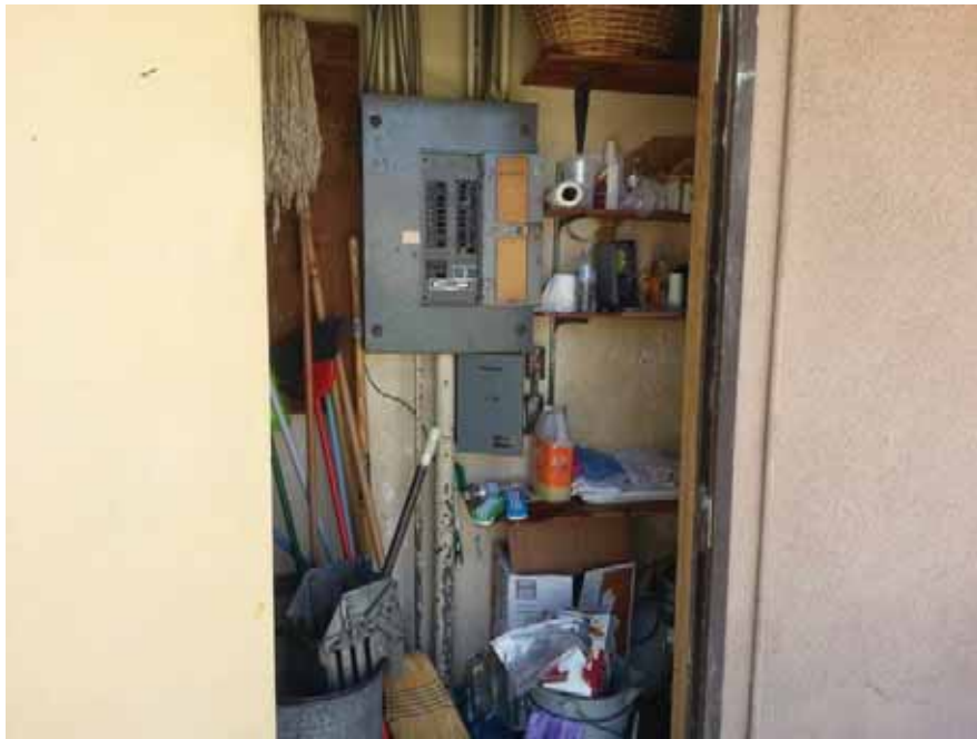
7. View of Janitor's Closet and Over the Counter Cleaning Chemicals at the Northwest Building.
