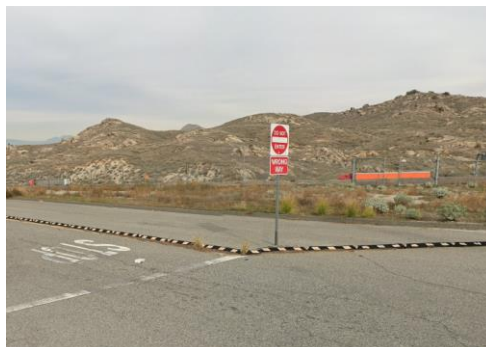
Figure 1: Rubber Curb and signage installed to modify circulation at Sycamore Canyon at El Cerrito
