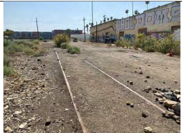
Railroad spurs to the north west side of the Property observed along parcel 211071023
