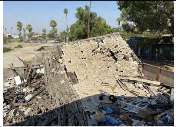
View of the portion of the building collapsed due to recent fire
