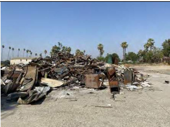
View of building material debris, scrap metal, and former concrete pit scale
