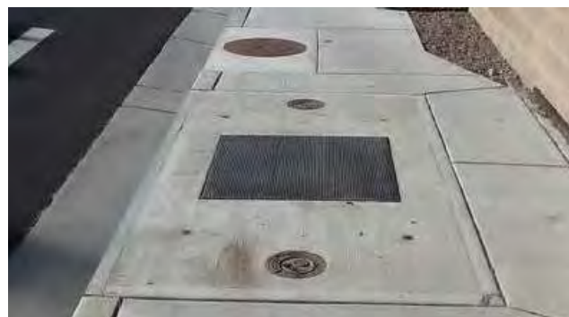
Figure 2b. Filterra with Full Grate Photo
