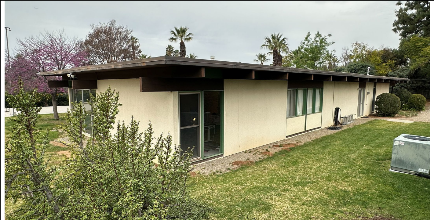
Rear and east side/rear elevation showing example of double-hung vinyl replacement of jalousie window in original opening, view northwest
