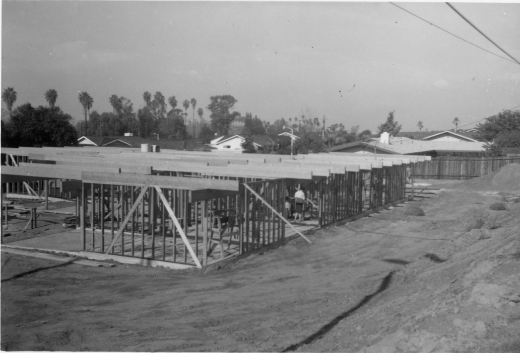
Edie under construction, showing rear/east side elevations and owner Mrs. Margaret Robinson and son Don touring the framed rooms, 1966
