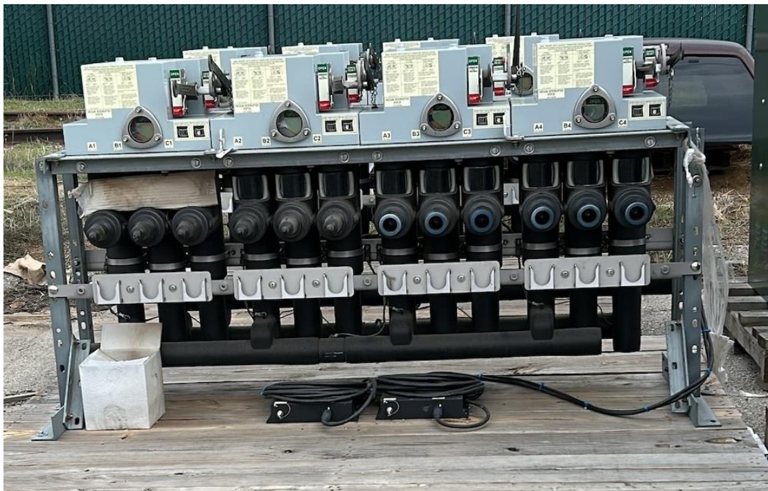
Typical Underground Switch
