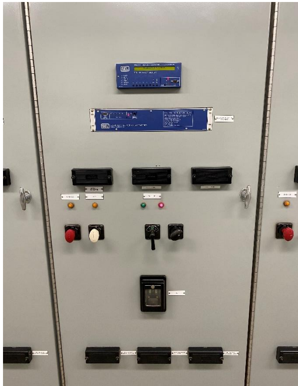
Typical 1 st Generation Digital Relays
