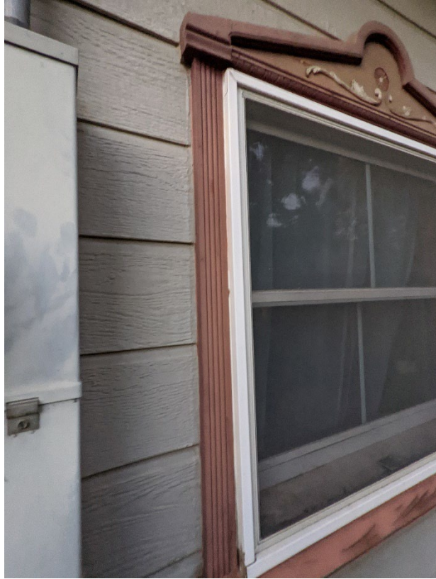
Figure 5 - Detail Photo showing modern siding, modern side window trim, and clad windows
