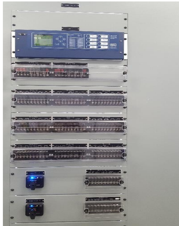
Typical New Digital Relays
