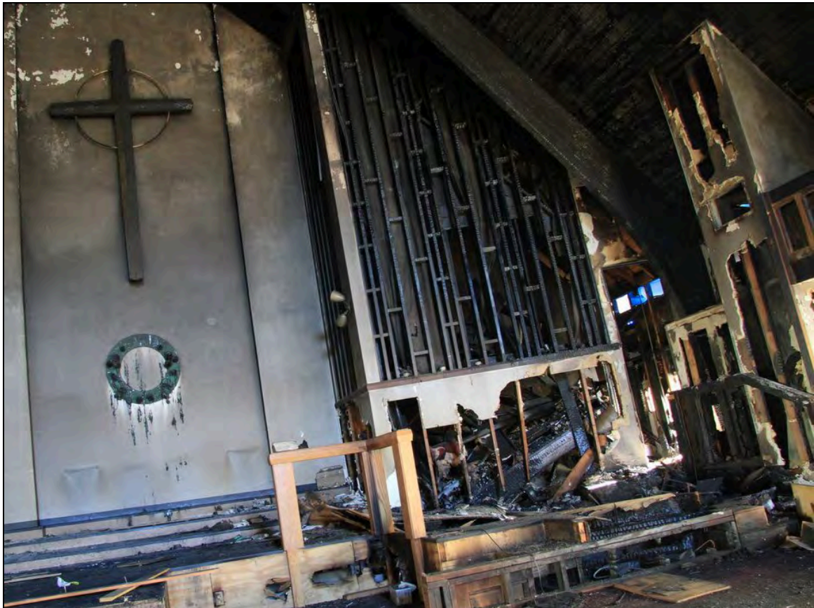
Magnolia Presbyterian 1965 Sanctuary Interior Fire Damage (December 2018)
