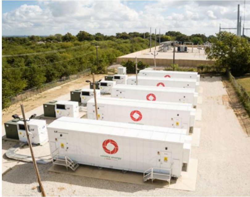
Figure 1: Battery Energy Storage Facility
