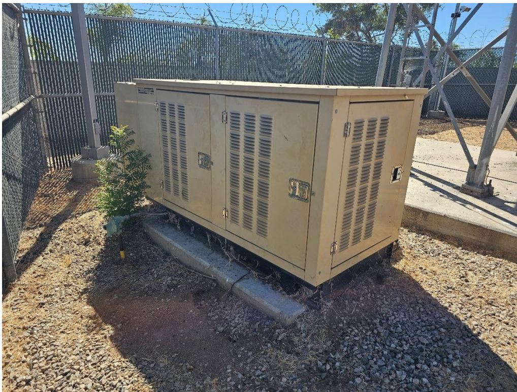
Existing Generator at Orange Terrace Radio Site
