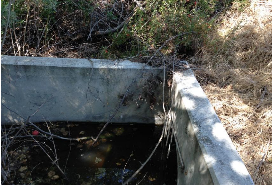
Photo 1 – Looking west at the 36-inch underground culvert that conveys nuisance flow from the adjacent residential development. This photo was taken in an off-site location.
