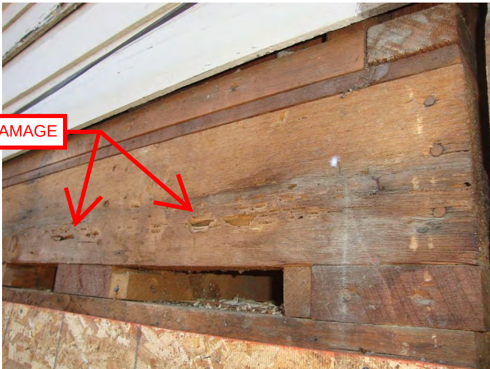
PHOTO 5: NORTH ELEVATION – DAMAGED RIM JOIST
