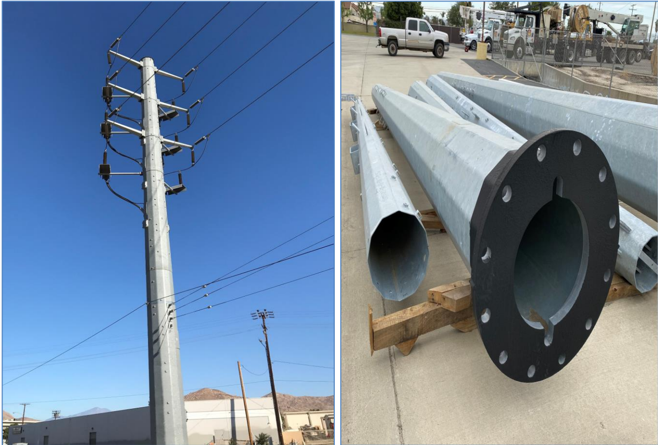
Tubular Steel Pole Structure
