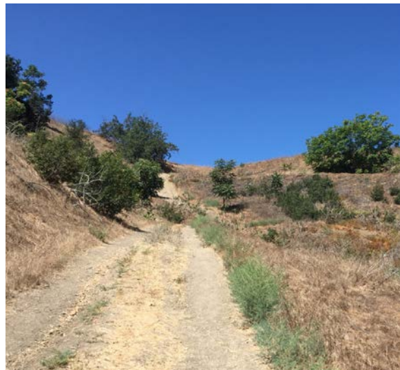
Long, straight sections of steep trail can lead to long-term erosion issues
