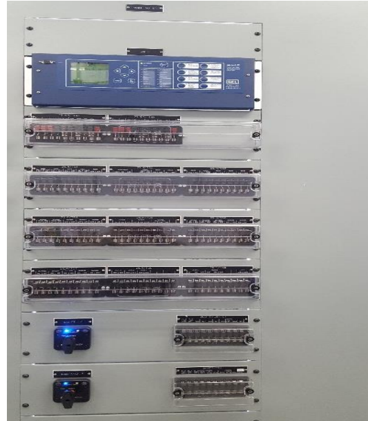
Typical Microprocessor Relays
