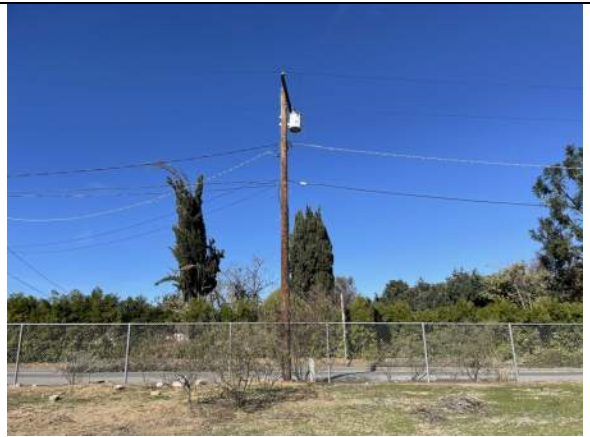
16. View of pole-mounted transformer along northwestern boundary of Subject Property
