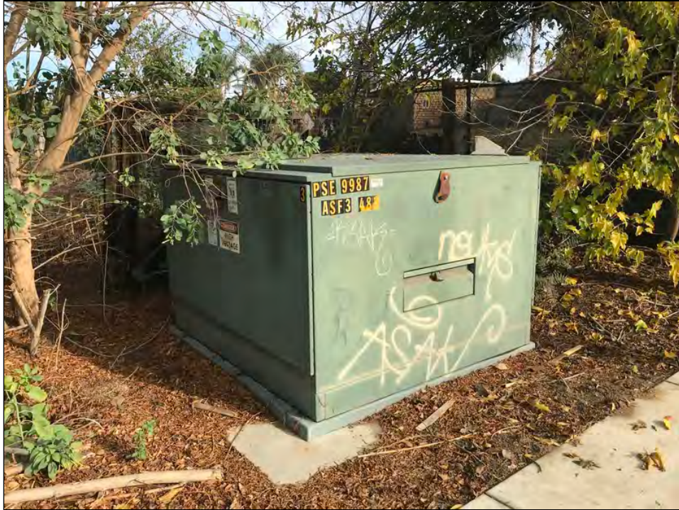
Photo 10: View of pad-mounted transformer.
