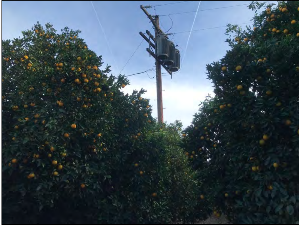
Photo 9: View of pole-mounted transformers.
