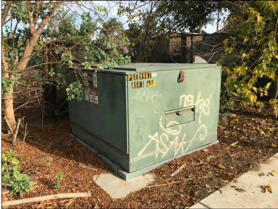
Photo 10: View of pad-mounted transformer.
