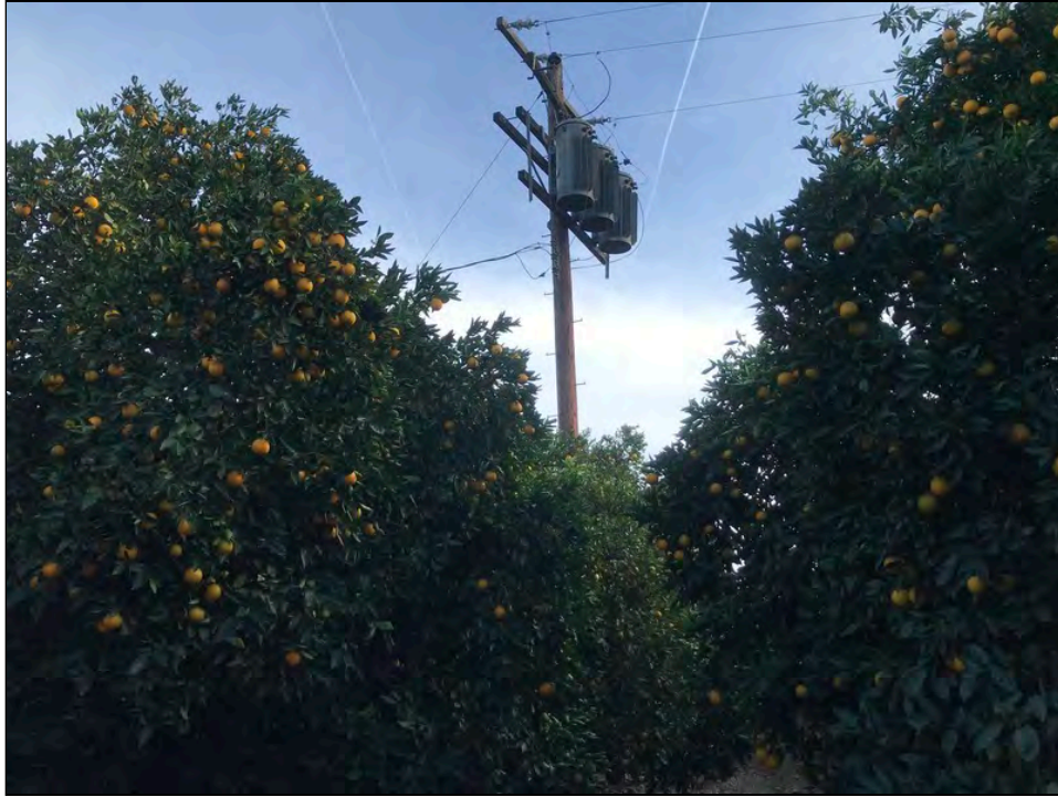
Photo 9: View of pole-mounted transformers.
