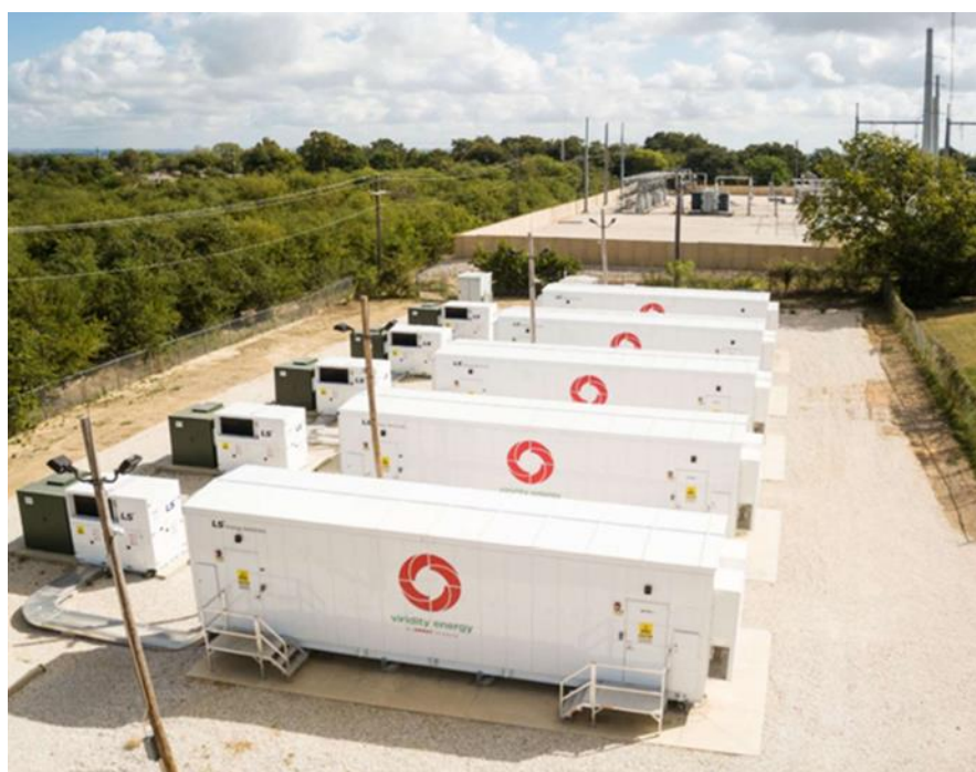
Figure 1: Battery Energy Storage Facility
