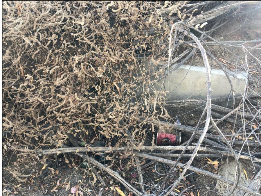
Existing headwall located at the upstream end of Unnamed Drainage A Tributary.
