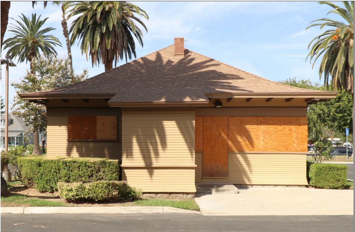
Photo 4. East elevation, view west (10/7/24). Fire damage was not evident on this rear elevation.
