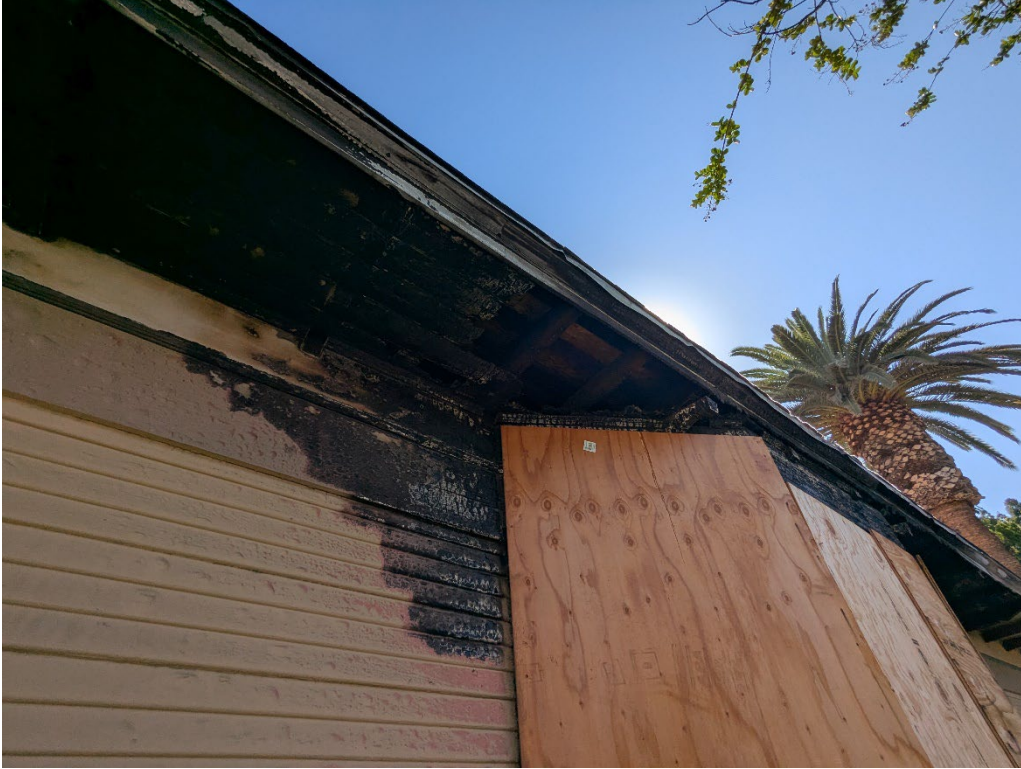
Figure 9 - South side fire damage
