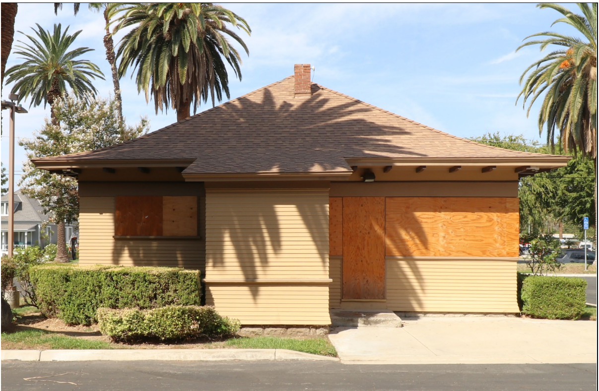
Photo 4. East elevation, view west (10/7/24). Fire damage was not evident on this rear elevation.
