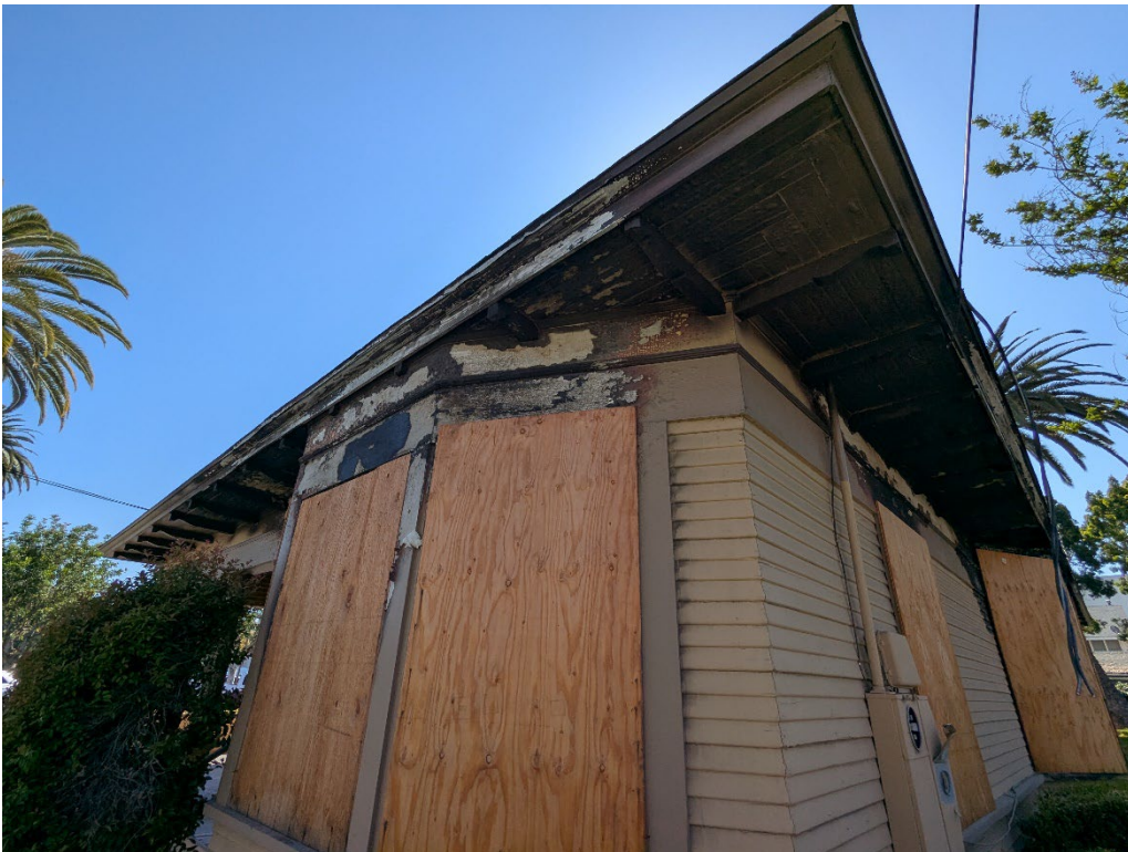
Figure 8 - Front and south side fire damage
