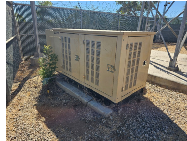
Existing Generator at Orange Terrace Radio Site
