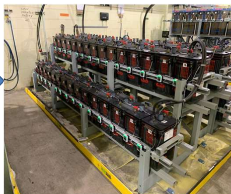
Typical Flooded Battery Bank (new standard)
