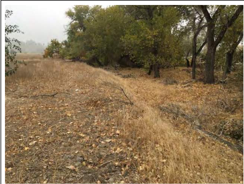
Photograph: 5 Photo Date: 12/2/21 Location: Feature 1 – Upper Santa Ana River, Tequesquite North Extension Direction: Southwest Comment: Looking at the top of bank of Feature 1.
