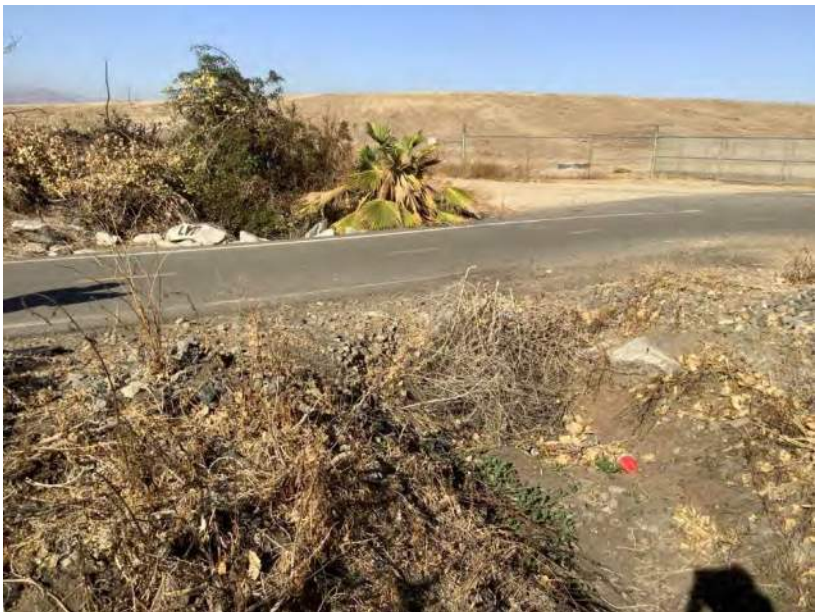
Photograph: 10 Photo Date: 12/2/21 Location: Feature 2 – Old Ranch Creek, Santa Ana River Greenway Direction: Northeast Comment: Looking downstream at culvert clogged with debris.
