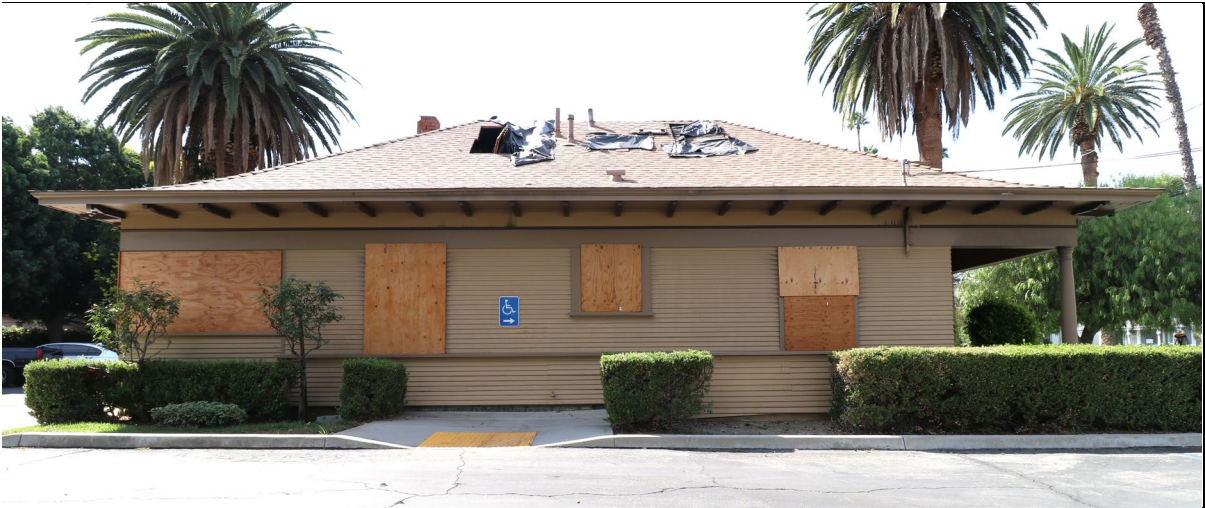
Photo 5. North elevation, view south (10/7/24). Note holes in the roof and minor evidence of fire under the eaves.
