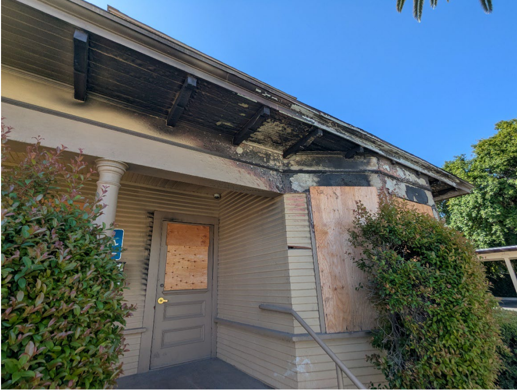
Figure 7 - Front facade fire damage
