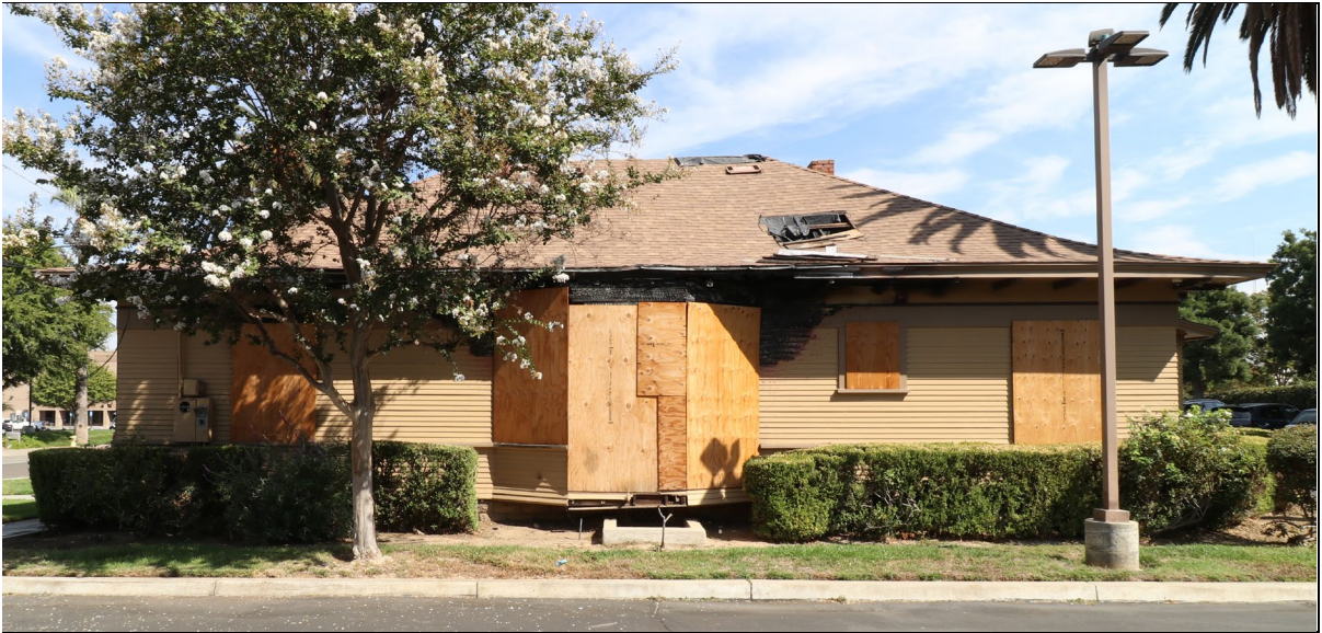
Photo 3. South elevation, view north (10/7/24). Note holes in the roof and charring along the eave and bay window.
