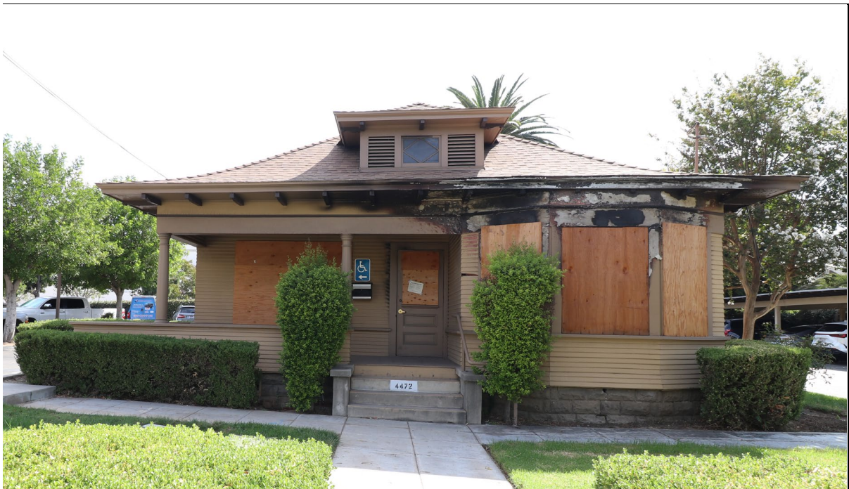
Photo 2. Façade, view east (10/7/24). Note fire damage above the porch and bay window.
