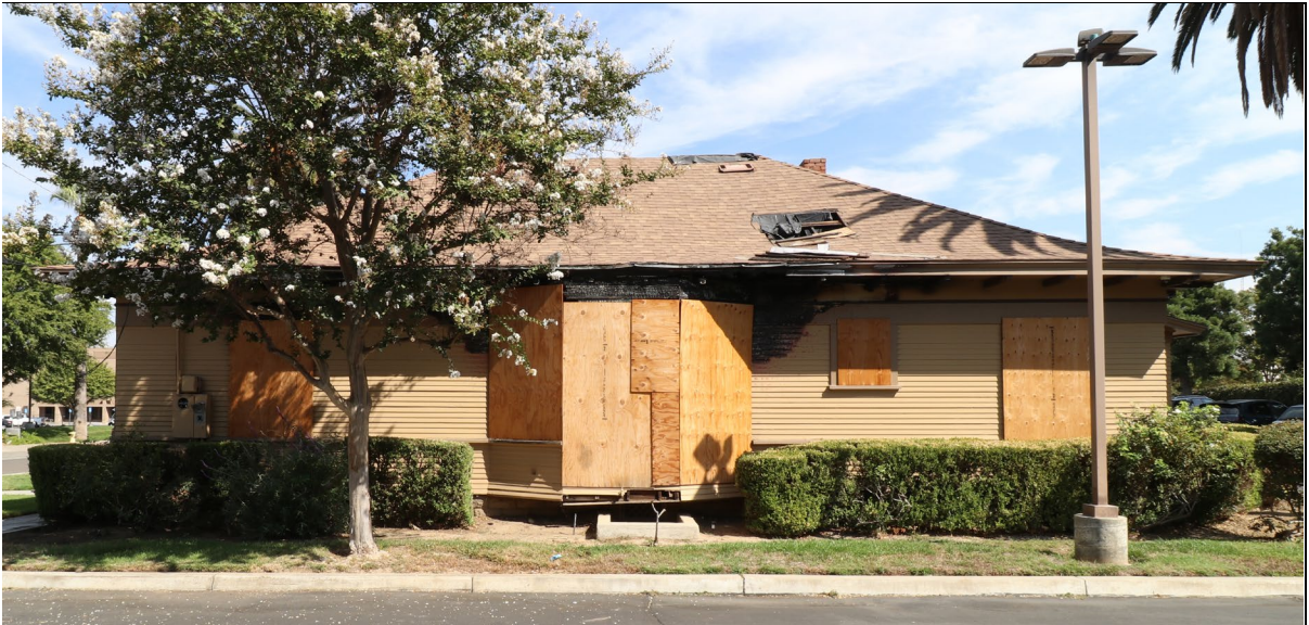
Photo 3. South elevation, view north (10/7/24). Note holes in the roof and charring along the eave and bay window.
