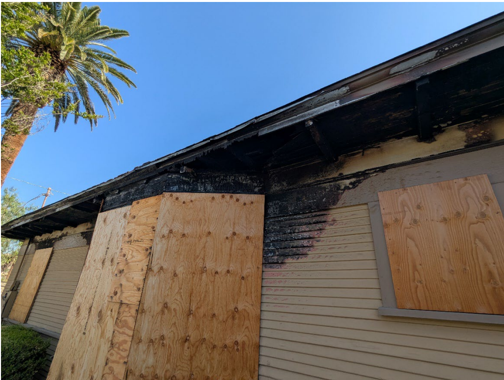
Figure 10 - South side fire damage
