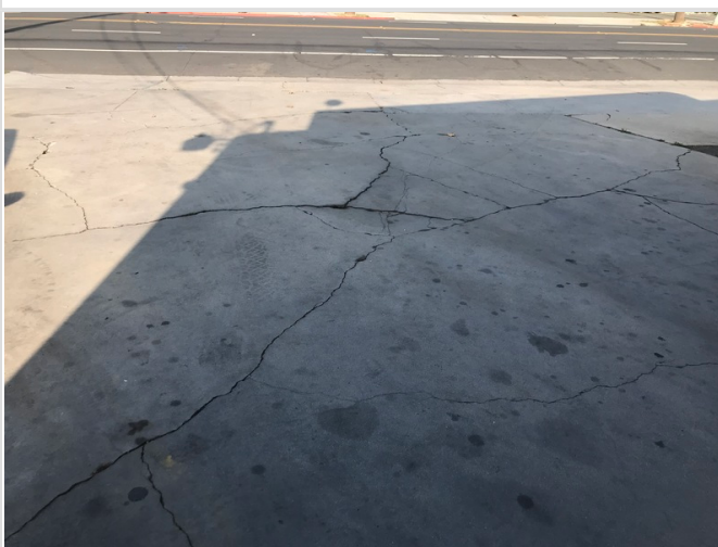
28. Minor staining on pavement
