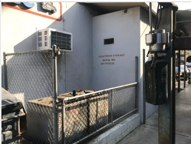
23. Hazardous materials enclosure
