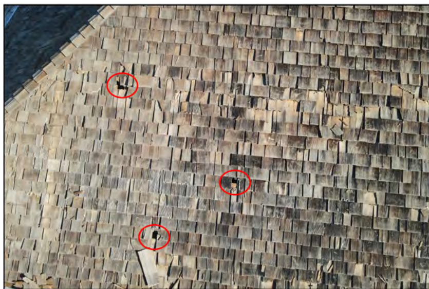
Harada House Main Roof South (ISA Site Analysis: Harada House Phase I)
