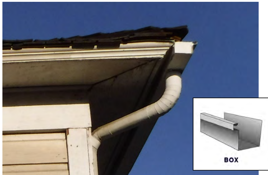
Existing Harada House Gutters and ca. 1960s-1970s Box Type Gutters (inset)
