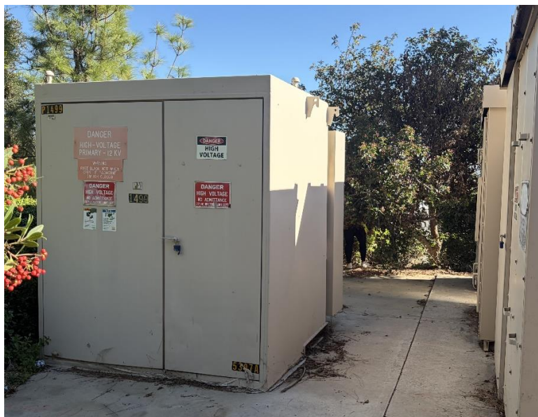
Existing Transformer to be Replaced
