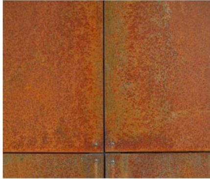
WEATHERED STEEL HUES OF RUSTED RED & BROWN OCCURS AT RESIDENTIAL - STREET CORNER FRONTAGES - ALL LEVELS, LOBBIES AND AMENITY AREAS
