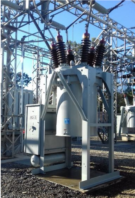
Typical Oil Circuit Breaker (Aged Unit)
