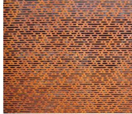
PERFORATED STEEL HUES OF RUSTED RED & BROWN OCCURS AT STAIR TOWERS - ALL LEVELS
