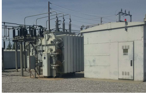
4kV Rated Equipment to Remove at Plaza Substation
